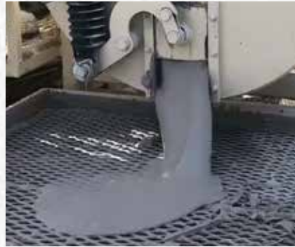
Clean mixer discharge
